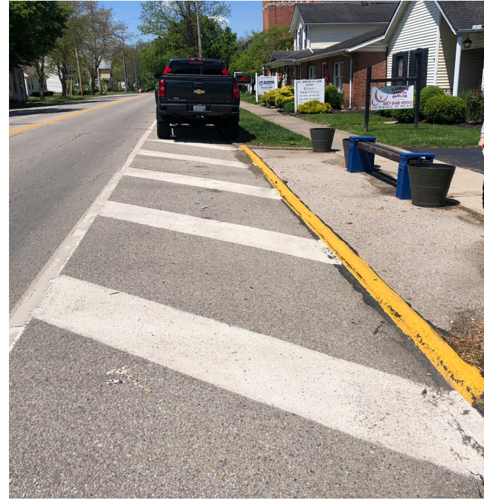
C. UNUSED CURB CUT
